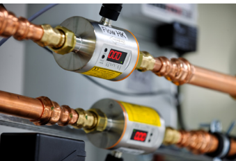
The test platforms used at NEXT ENERGY are fitted with extensive measuring equipment for CHP system characterisation.
