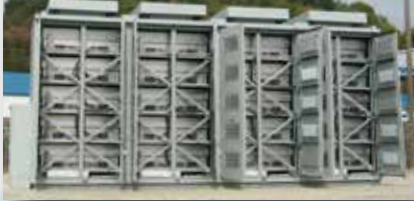
1,000 kW (6,000 kWh) NAS system for Chemical Station, WV
