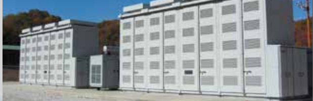
2,000 kW (12,000 kWh) NAS system for Balls Gap, WV
