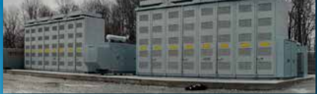
2,000 kW (12,000 kWh) NAS system for East Busco, IN
